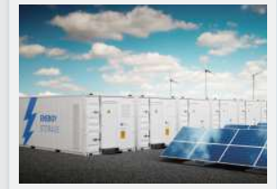
Energy Storage System (ESS)
