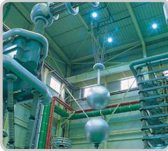
High Voltage Test / Impulse Test
